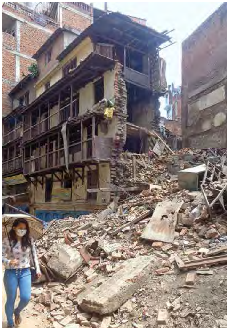
A collapsed building in the historic city of Kathmandu
