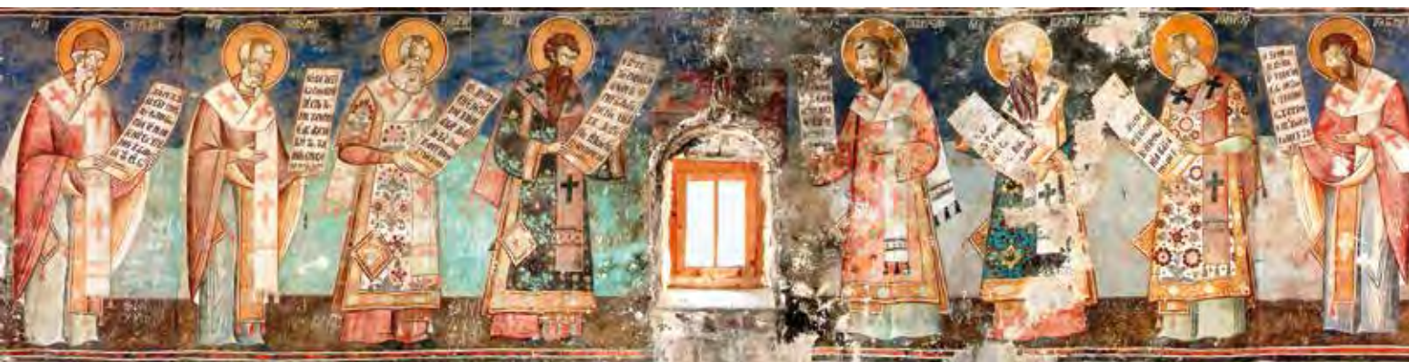
St. Athanasius Church, lower register of the apse, degradation of the paint layer
