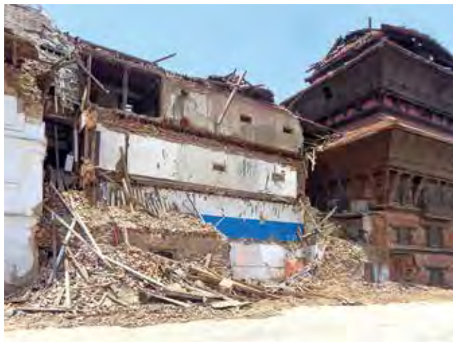
Collapsed structures of the Hanuman Dhoka Palace Museum, Kathmandu
