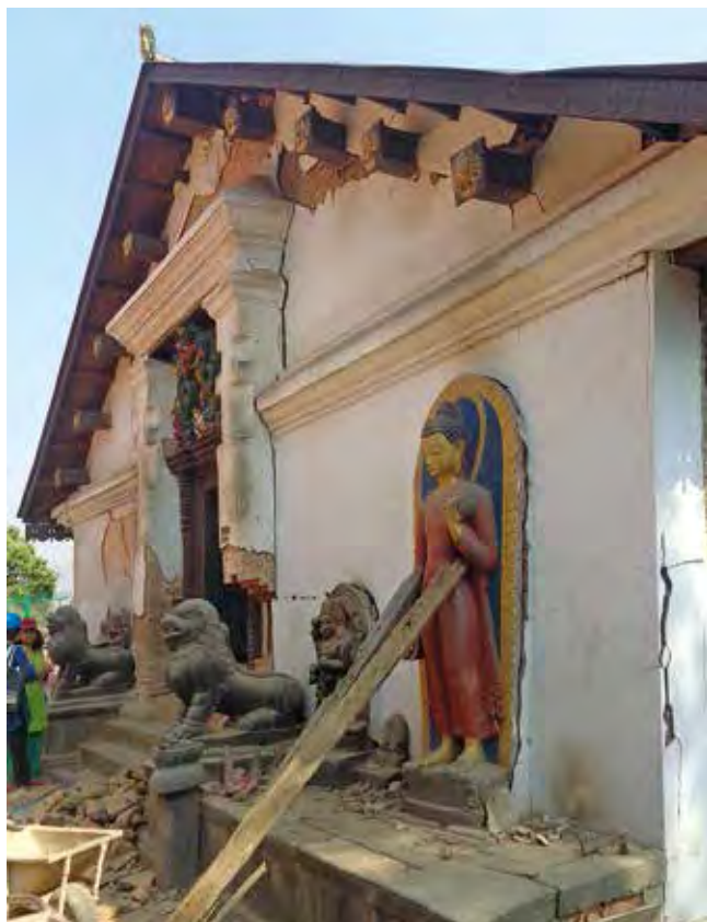
The damaged entrance to Shantipur, the tantric temple, which can only be entered by an initiated priest
