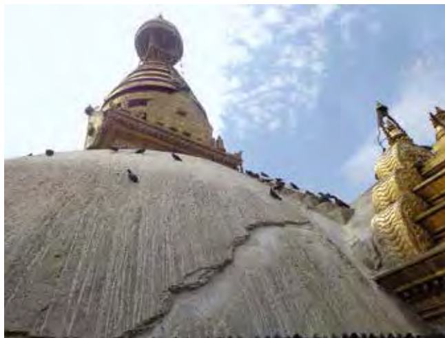
The Swayambhu Mahachaitya showing the temporarily sealed cracks after removal of layers of lime-wash
