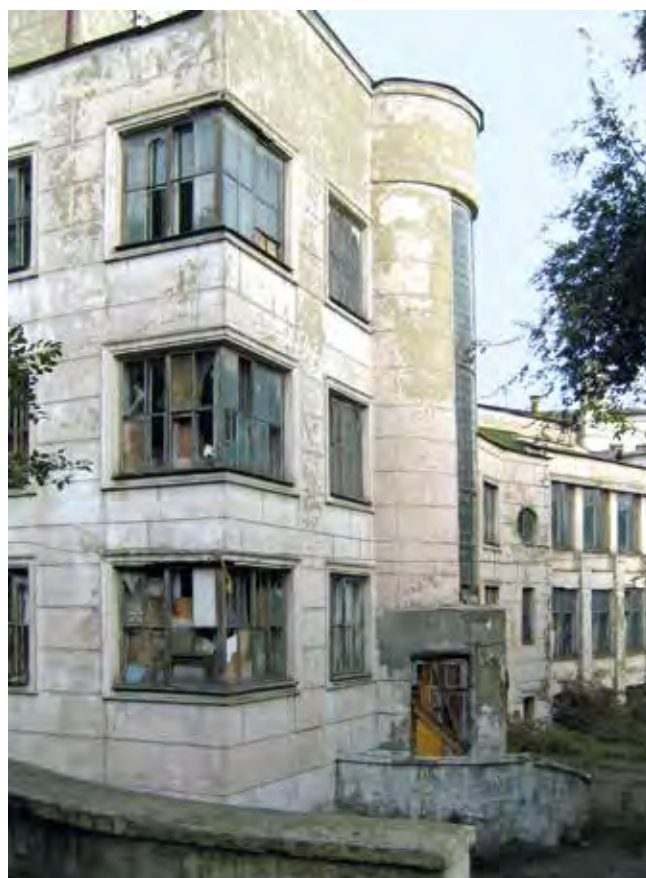
Former Metalworkers' Palace of Culture in Dnipro, condition in 2011 (photo S. Smolenska)
