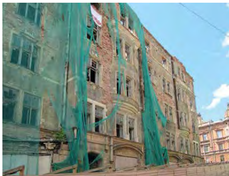
Krepostnaja uliza 3 built in 1904; the last inhabitants left 25 years ago (photo Maija Kairamo 2013)
